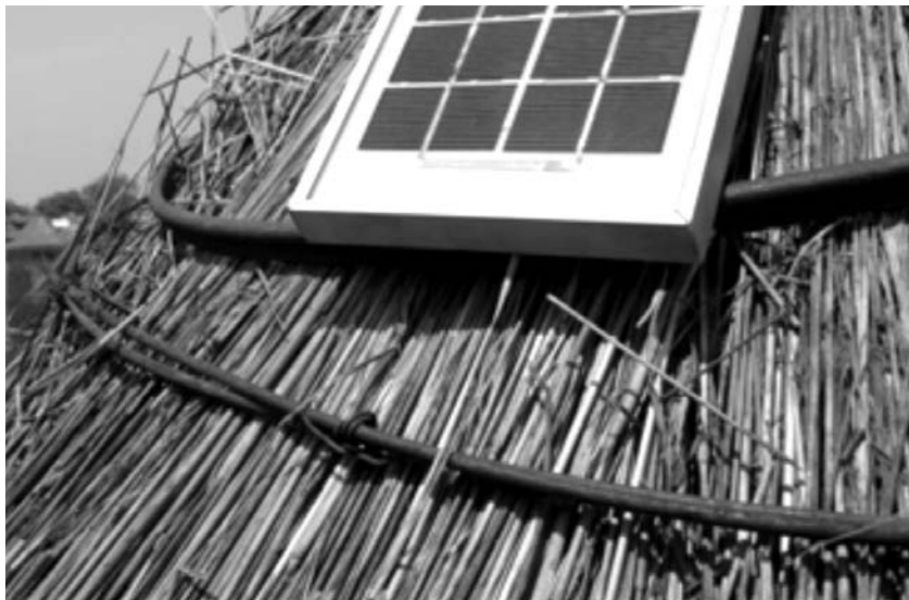
Off-grid solar system. 24
